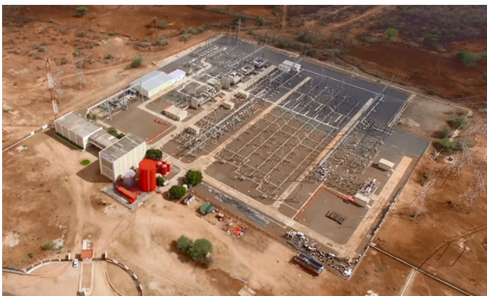
Photo of Matambo substation in Tete
